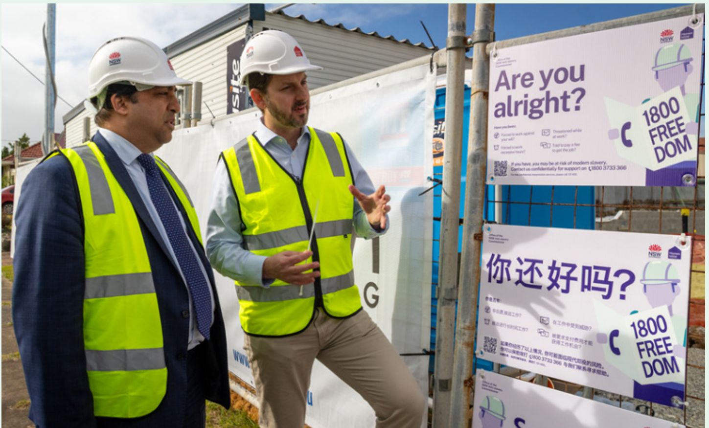
Naveen Chandra, Executive Director, Housing Portfolio, Homes NSW and Dr James Cockayne, NSW Anti-slavery Commissioner, visit a Homes NSW construction site in Newcastle where new signage promoting 1800 FREEDOM is displayed.
